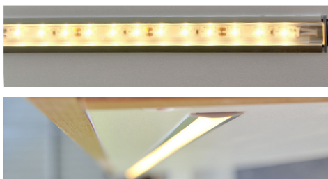
Images of Lighting Installed
